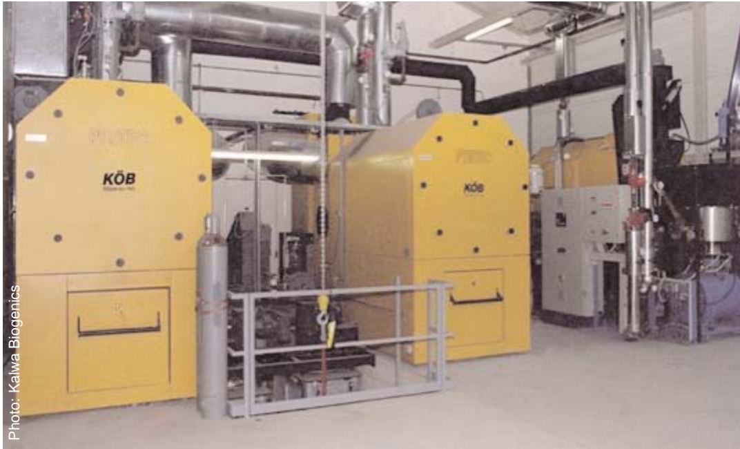
One of the cogeneration heating systems installed by Kalwa Biogenics of Edmonton
